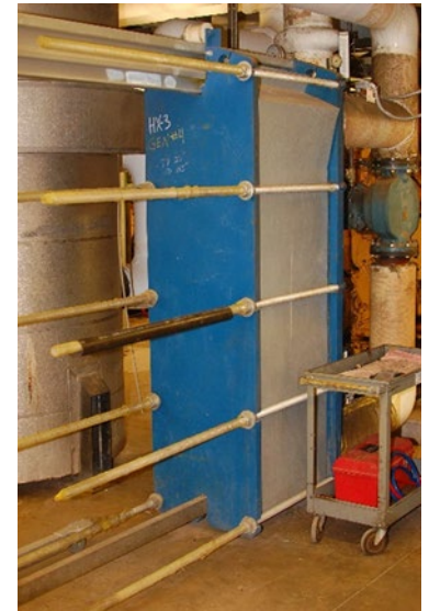
A plate & frame style heat exchanger capturing the heat from one of the gensets.
