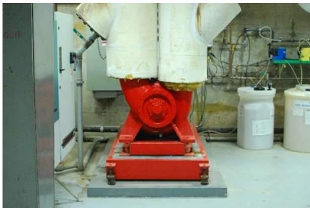
One of the pumps that circulates hot or chilled water through the buildings.
